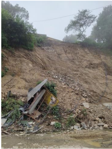
(g) Agrakhal landslide
