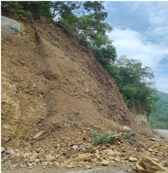
(c) Belta 1 landslide
