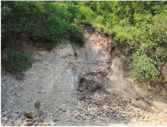
(a) Jhaki Dagar 1 landslide
