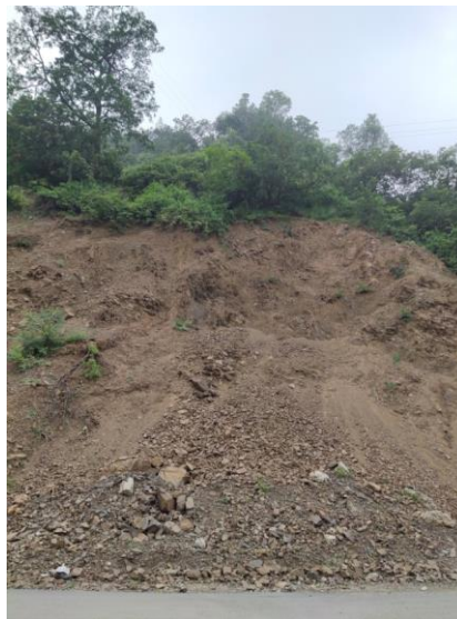
(i) Pildi landslide
